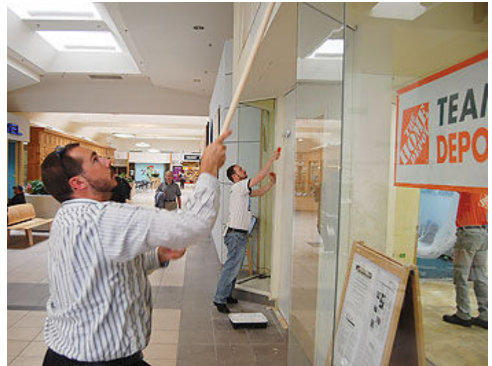
Niles Teen Center Supervisor Sean Miller (left) paints high as Teen Center Director Mark Williams (background) paints low during Teen Center expansion work Thursday at Golf Mill.
